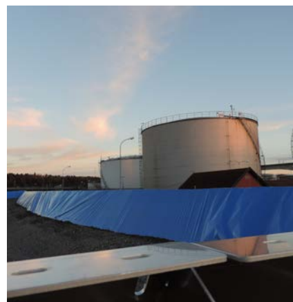
Photo shows the barrier H180 from the water side.
